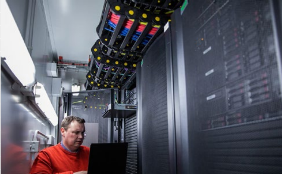
The RSA data centre located at Ballina headquarters
